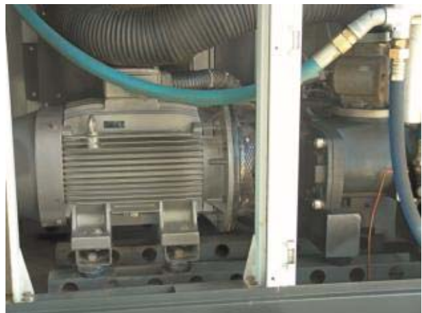
Figure 6. Compressor with PM motor
