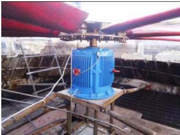
Figure 10. Cooling tower with PM motor
